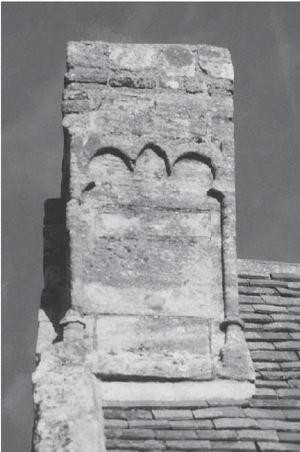
Fig. 11.27 The Court Hall, Quarter 8. Medieval chimney cap showing the cusped head to the recess and the attached corner shafts in the south face.
