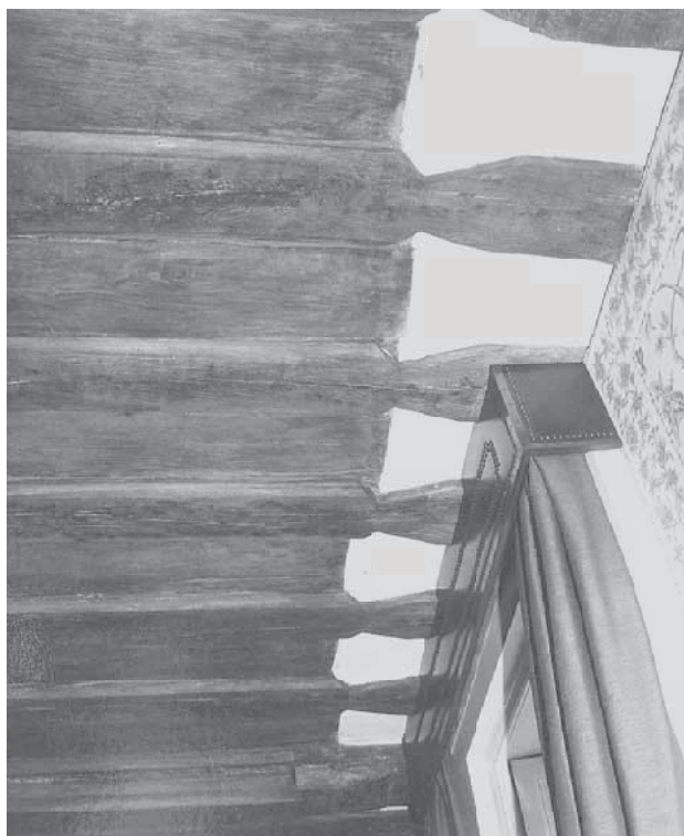
Fig. 11.14 Periteau House, Quarter 7. Ceiling joists to the ground-floor room showing the boarded ceiling and dovetails on every joist to accommodate the former jetty plate.
