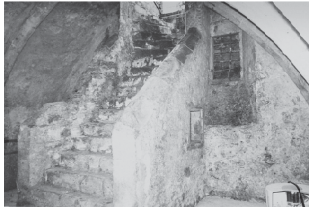
Fig. 9.21 Cellar 26. The parapeted handrail flanking the main entrance stairway projecting into the cellar. Note the original gridded window to the right.
