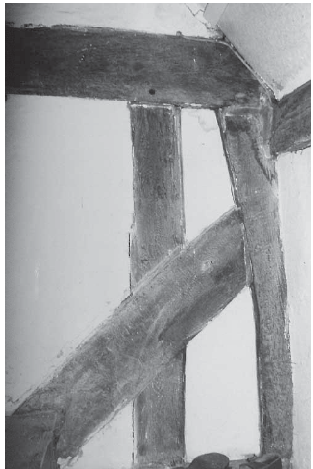
Fig. 11.9 The Retreat, Quarter 6. Inset post for Wealden front with a footbrace halved across the face of the post.
